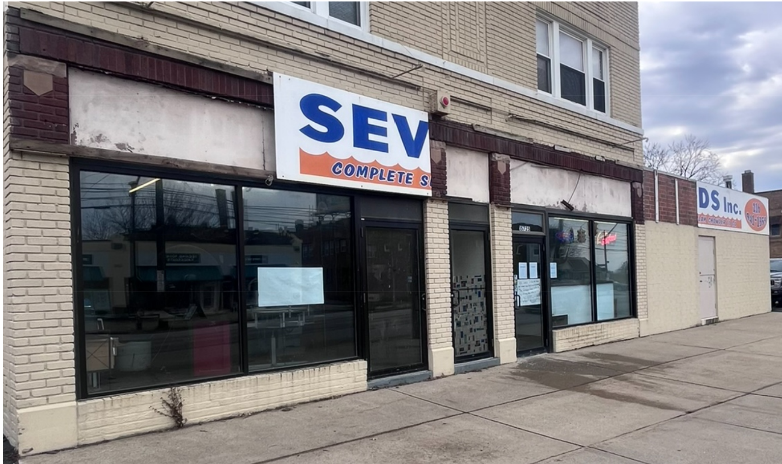
Existing Sign (showing damage due to high wind)
